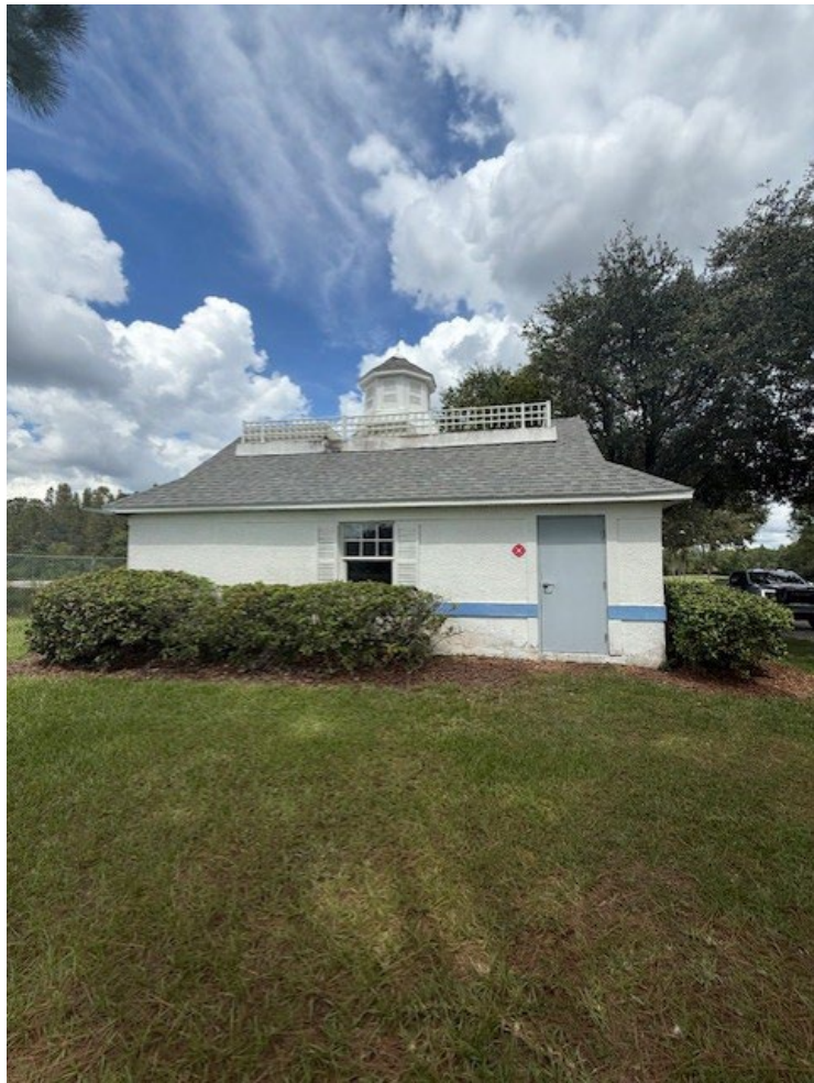
Pump House Next To Driving Range
